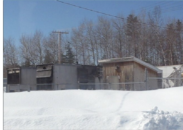
Illustration 8: Diesel generator for the entire community
